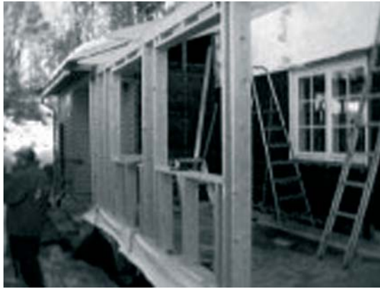
Figure 11 An MMS photo taken by a carpenter and sent to an architect to check on the details of a construction situation
